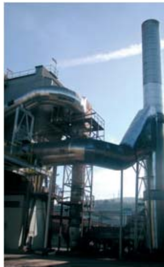
Gases Leaching System
