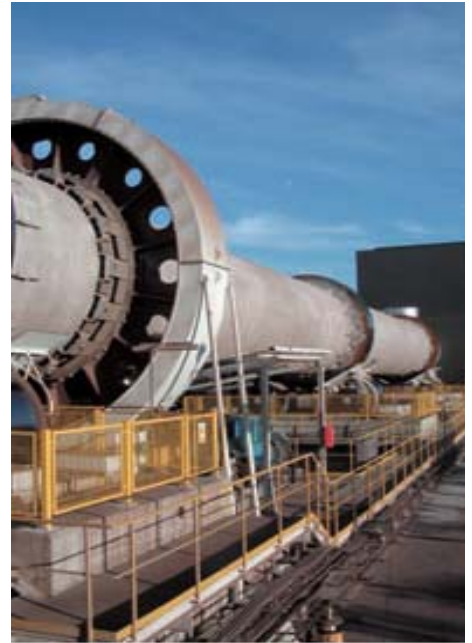
New Waelz furnace
