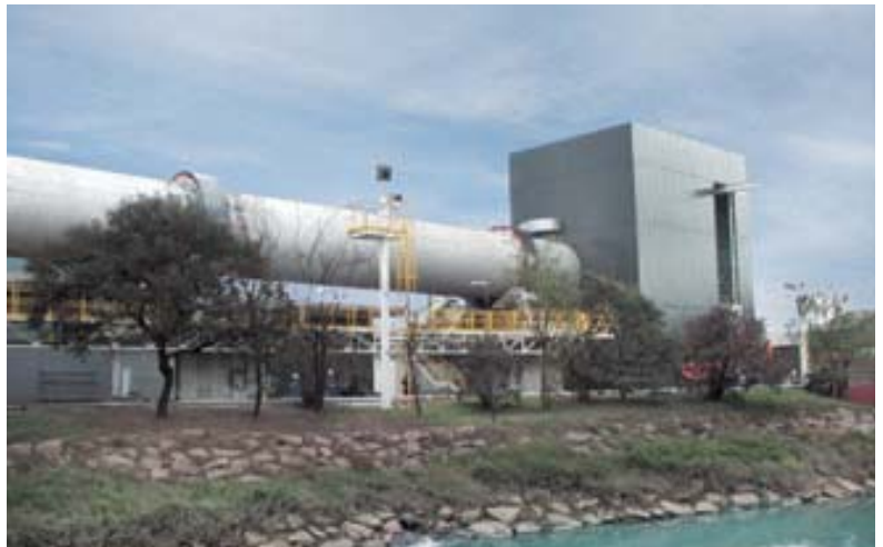
New Waelz furnace
